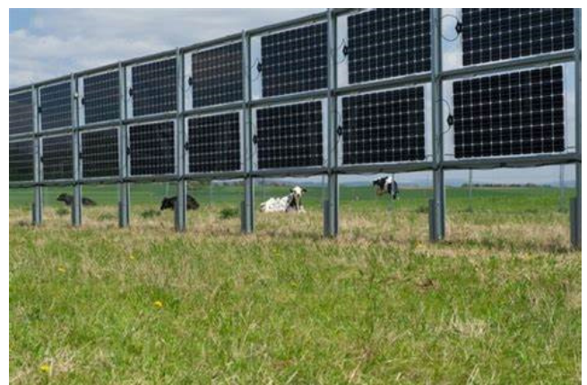
Verticale zonnepanelen in Culemborg
